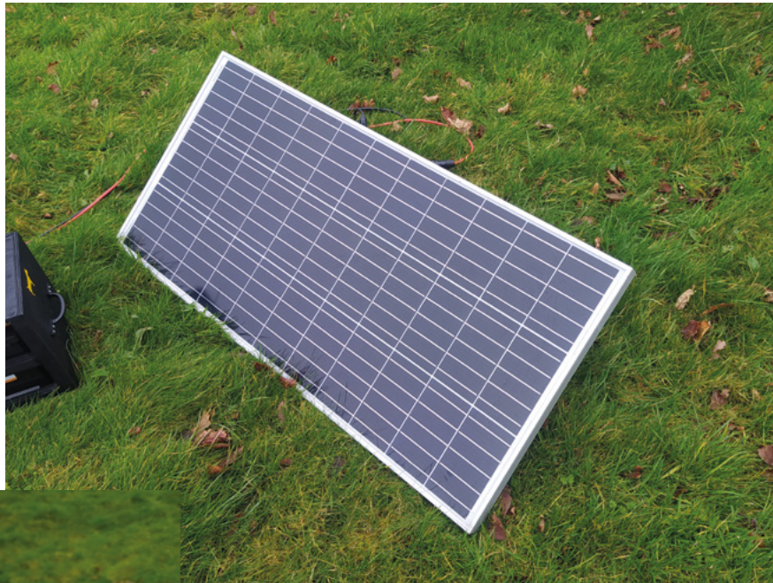
Figure 3 ↗ The MPPT charge controller receiving 1.7 A from the solar panel
