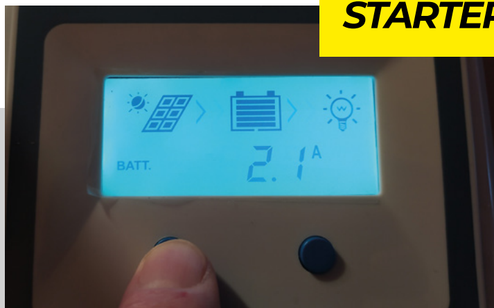
Figure 4 ♦ The MPPT charge controller having performed a DC-DC conversion is putting out 2.1A at 14.5V to the battery
