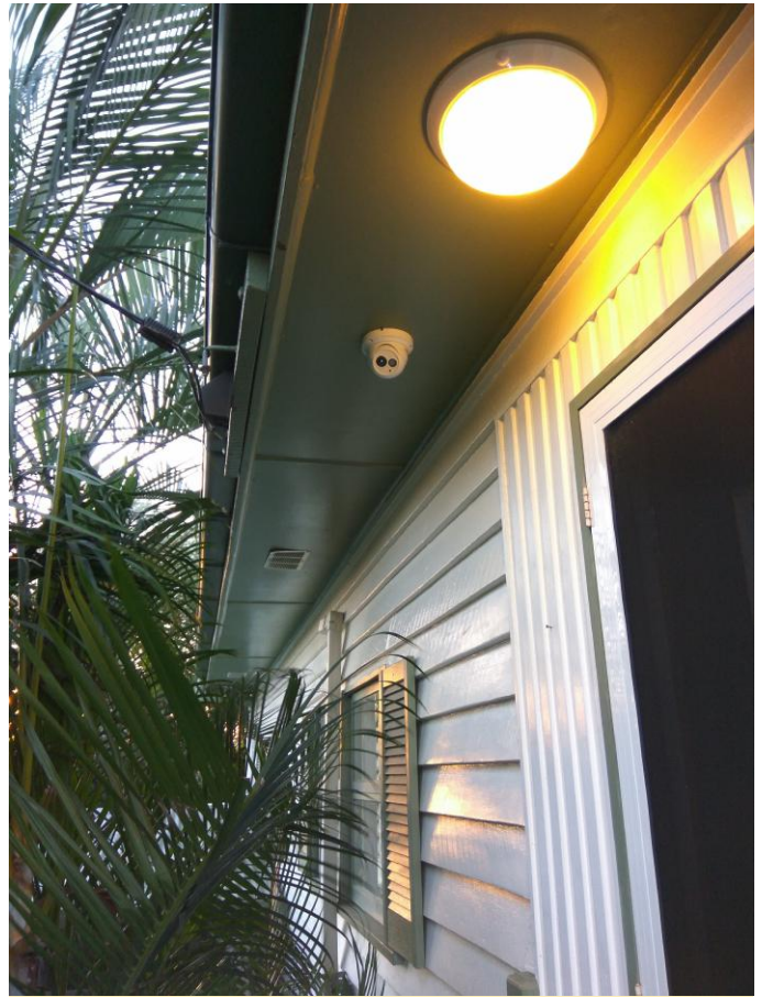
Figure 3 - Example Camera Install
