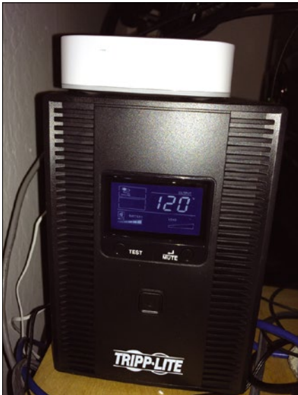
Figure 2: The SmartThings hub (top) and the emergency power supply for the Internet connection.
