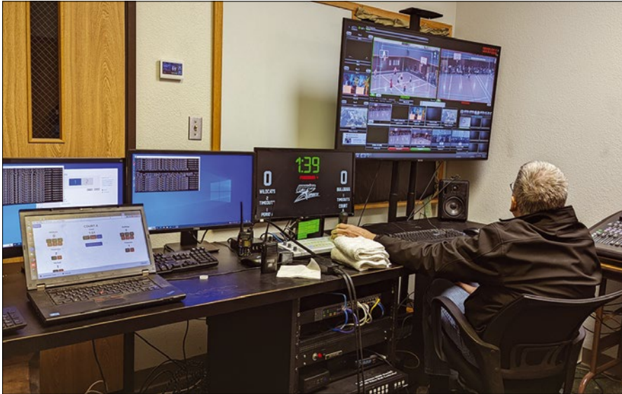
Figure 2: The video control room is a converted classroom. From left to right, the first two monitors in the background are the main displays of the NUCs running the scoreboard software. The text window is the output of the Python program, and the scoreboard itself is on the secondary monitor output. The third monitor is routable from the video matrix to select what is shown. In the foreground are the matrix control touchscreen and the camera controller. The tall monitor is the switcher multiview. The NUCs and the matrix are visible at the very bottom of the rack under the table.
